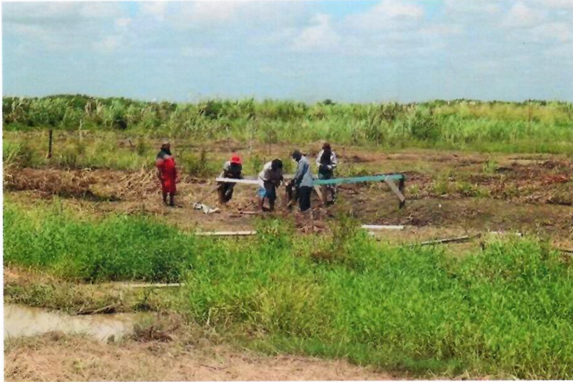
Squatters illegally constructing a structure on the GuySuCo land at Success ECD
